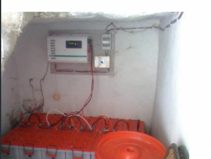
Inverter and battery system from Lotus Energy
