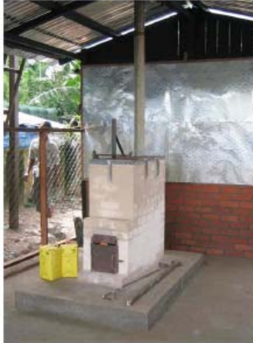
Figure 1.12. The Montfort Incinerator Mark8a [9]
